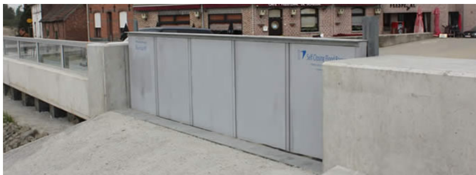
Figure 4: SCFB in operation
